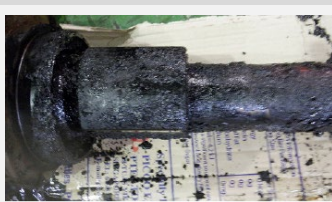
FUEL PUMP SUCTION VALVE FAILURE
